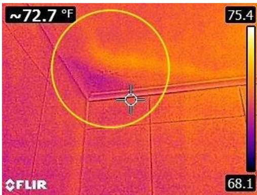
Photo 8-3 THE INFRARED SCAN SHOWS A TEMPERATURE ANOMALY INDICATING MOISTURE IN THIS AREA.
