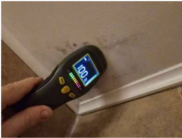
Photo 8-1 THE MOISTURE METER SHOWS ACTIVE MOISTURE IN THE CEILING AT THE TIME OF THE INSPECTION.
